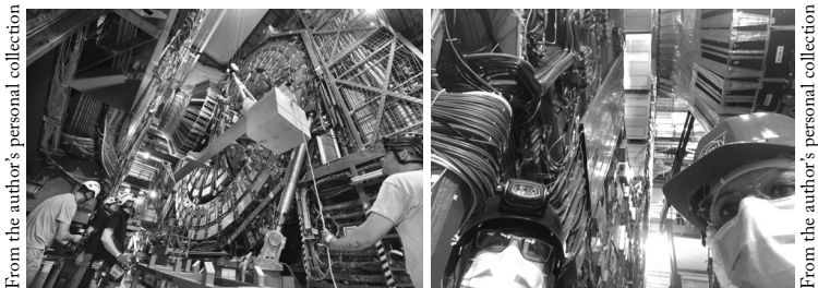
Left and Right: Commissioning of the newly installed GEM stations by my team, 2021
